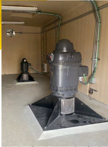
Interior of new pump station showing large and small capacity pump.
