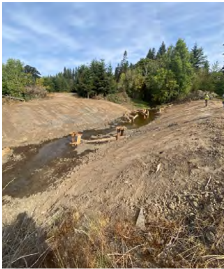
Lower end of restored Chicken Creek prior to installation of the new pedestrian bridge. This is the location of the former water control structure, located just east of the photo blind.
